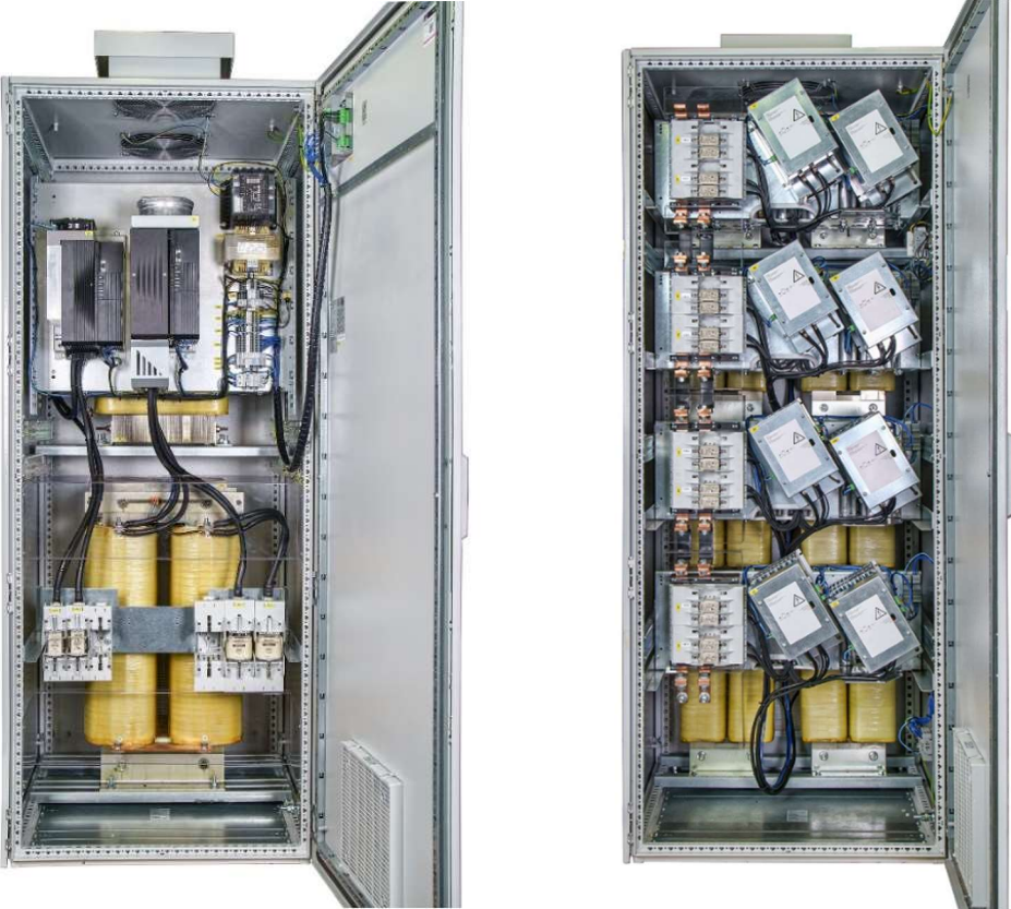
Photo 3. Systems for inductive and capacitive reactive power.
